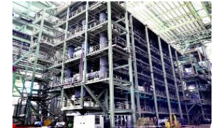
Hot Dip Galvanizing Lines (HDGL)
