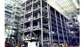
Hot Dip Galvanizing Lines (HDGL)
