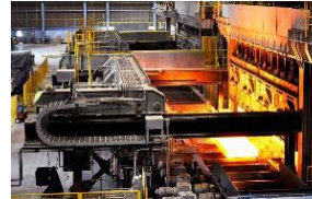
Hot Strip Mill (HSM) State-of-the-art HSM designed to roll AHSS, Line Pipe, & Stainless products
