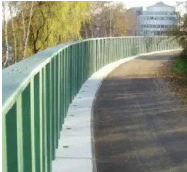
Flood protection barriers
